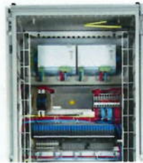
Cabinet System Solutions
